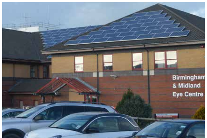
Solar PV panels on BMEC at City Hospital
