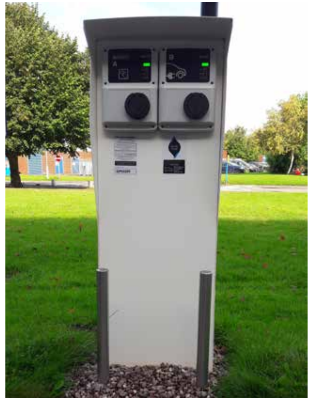
One of the Electric Vehicle Charge Points at City Hospitals, which have been introduced across our Trust sites.
